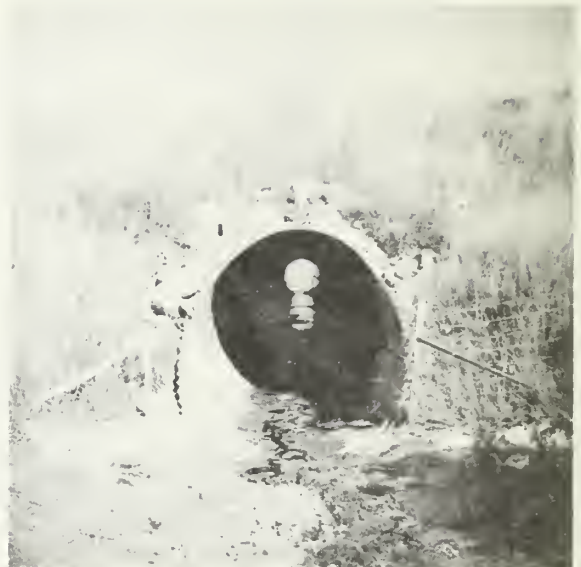
SOUTH ENTRANCE Notice drainage
